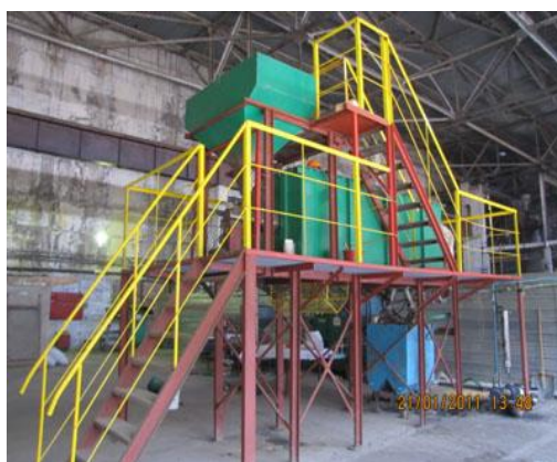
Figure 1. The pilot plant for the thermal treatment of RH
